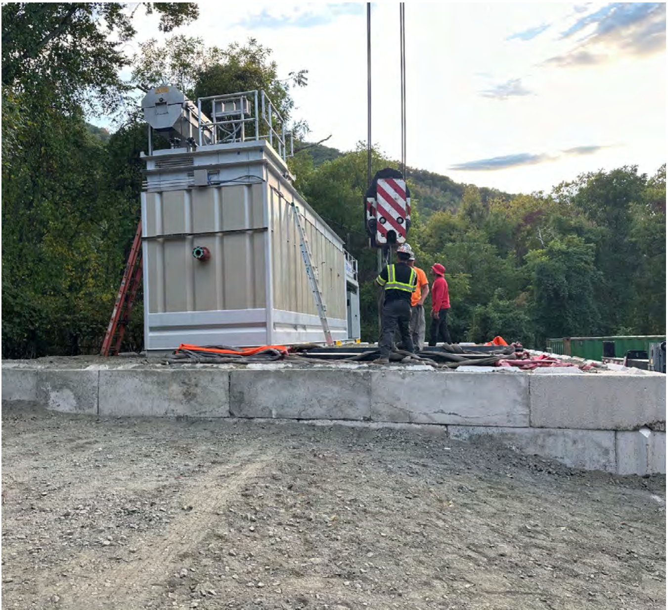
Delivery of Treatment Plant for Hot Springs in October, 2025.
