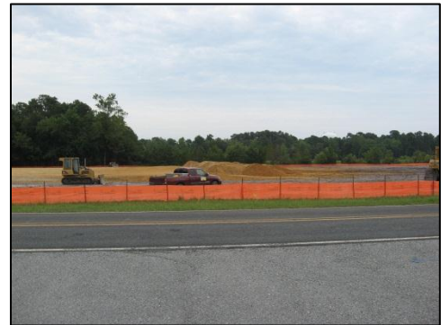
Preliminary site work for the construction of the GTP-7 shell building began in June 2011.
