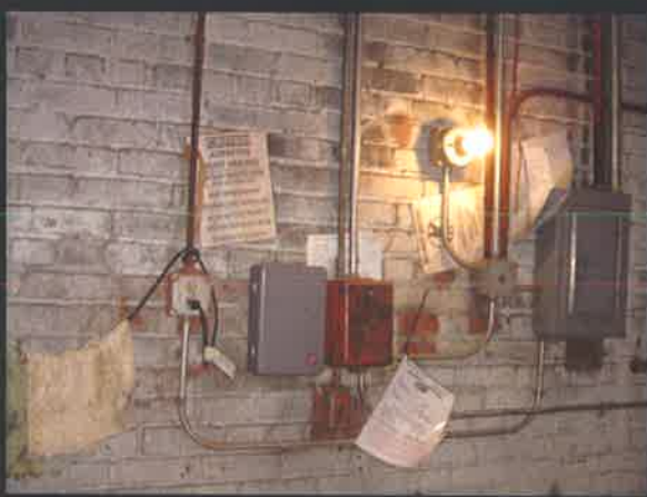
Deteriorating wiring in this boiler room poses a severe health and safety threat.
