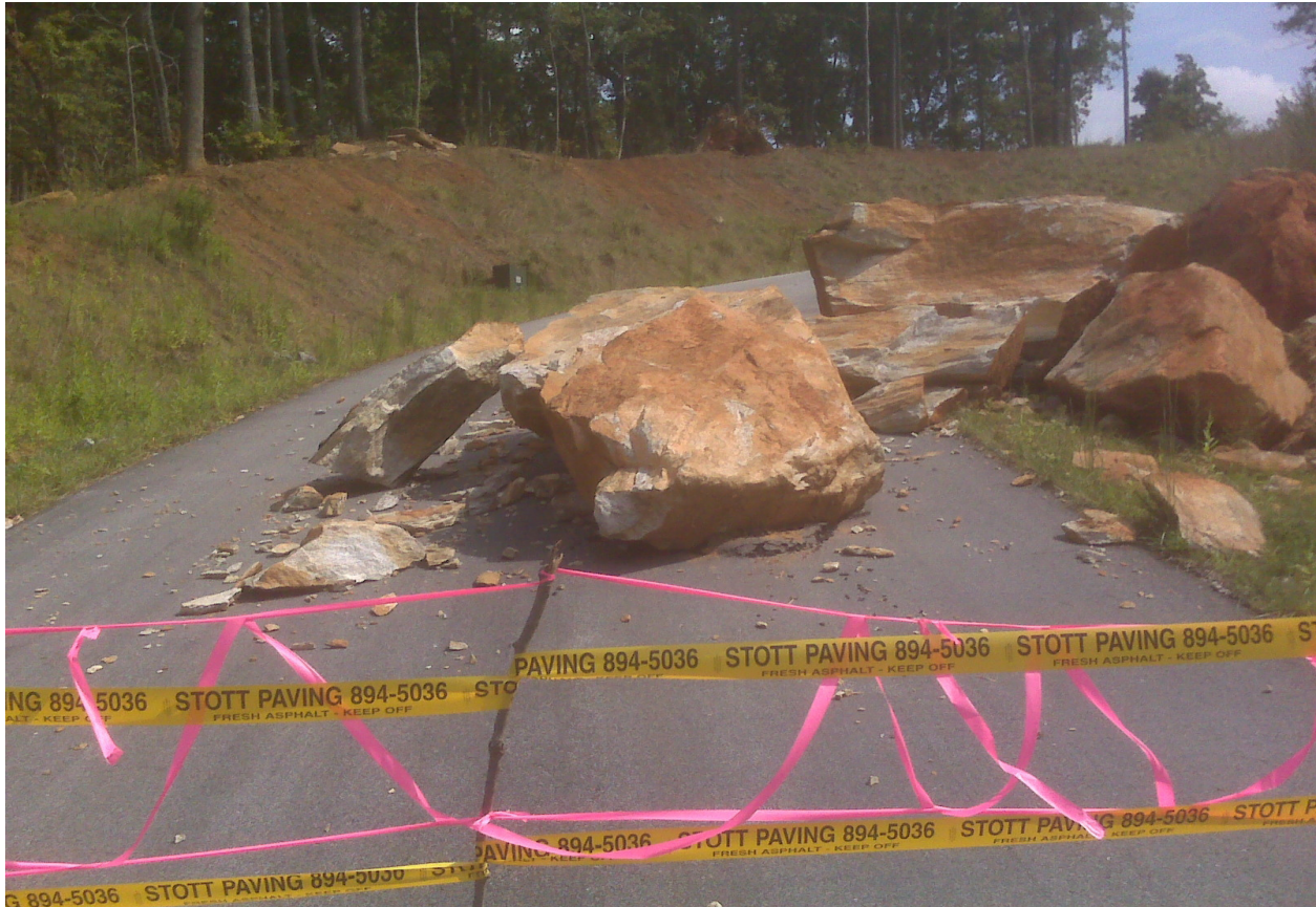
Rockfall at a Subdivision in Polk County.
