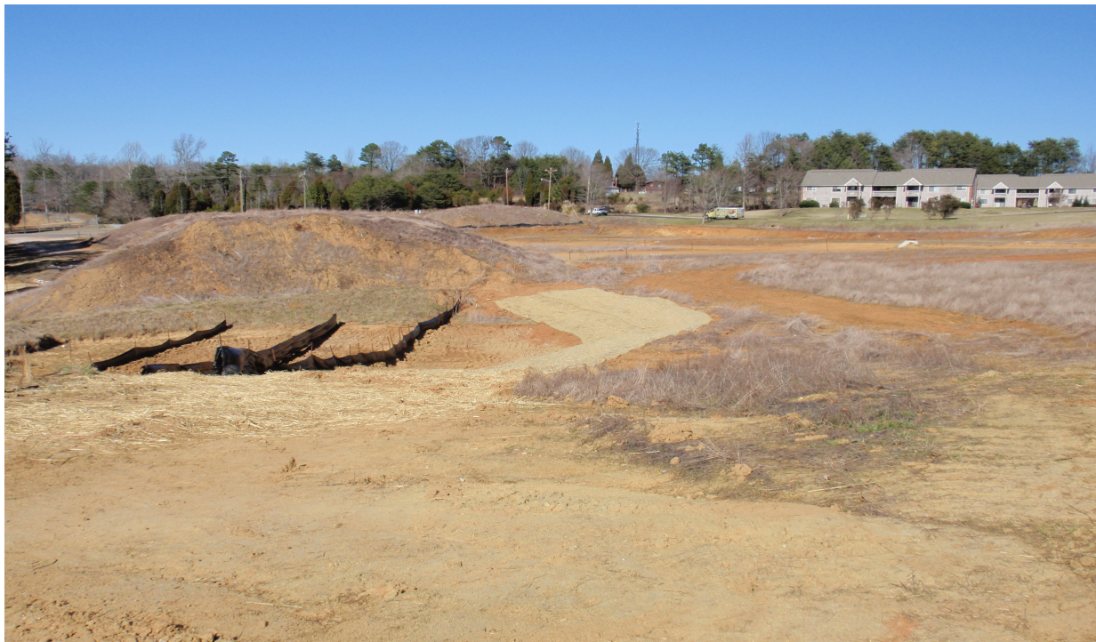
Foreclosed site in Rowan County with remedial measures provided by lending institution.
