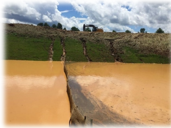
Figure 11 - Rill Erosion on Sediment Basin Slope
