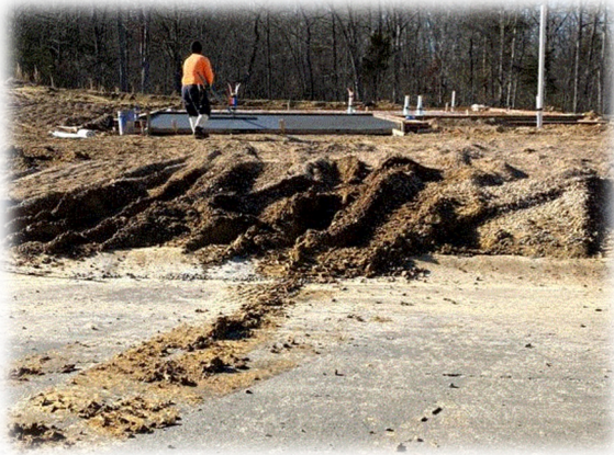
Figure 8 – Poor Construction Entrance
