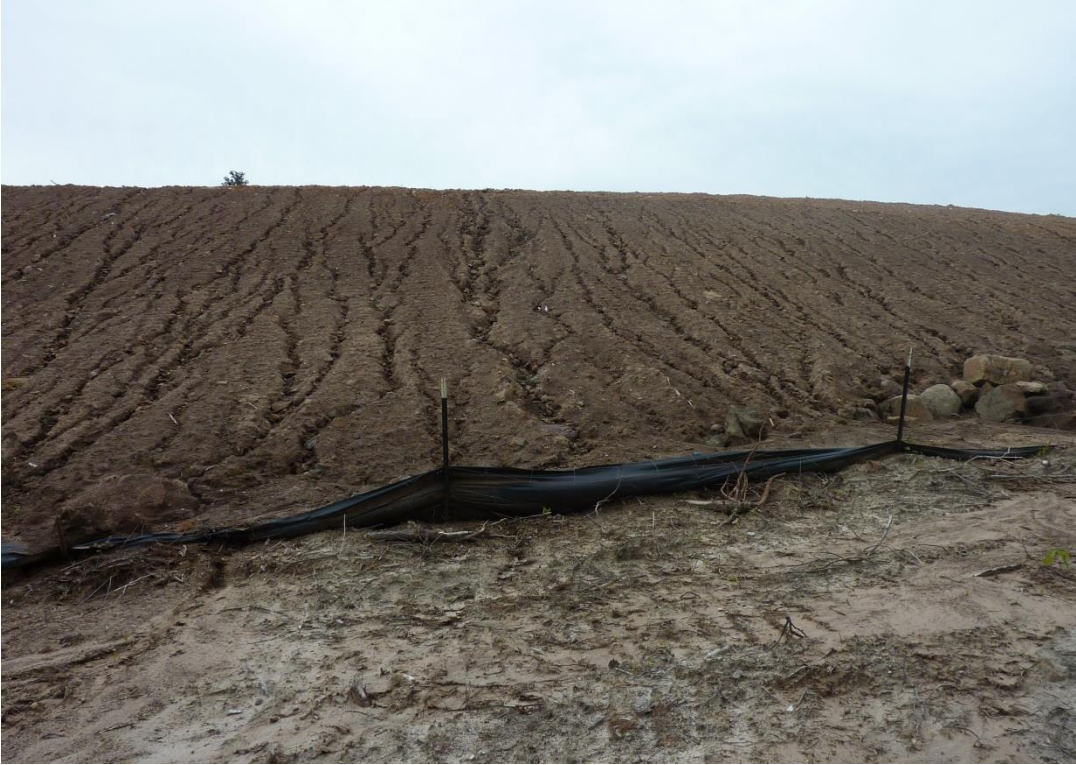
Bare, Eroding Slopes with Insufficient Measures to Prevent Sedimentation
