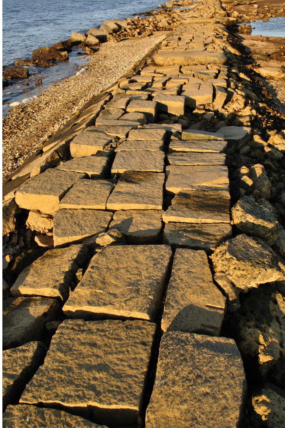
Figure 3. Photograph taken 12.11.2015 on the New Inlet Dam at low tide depicting a more intact portion of the dam surface. Photograph is for informational purposes only to support the Request for Information per 2015 Appropriations Act Section 14.6.(h) and does not necessarily represent conditions along the entire length of the New Inlet Dam.
