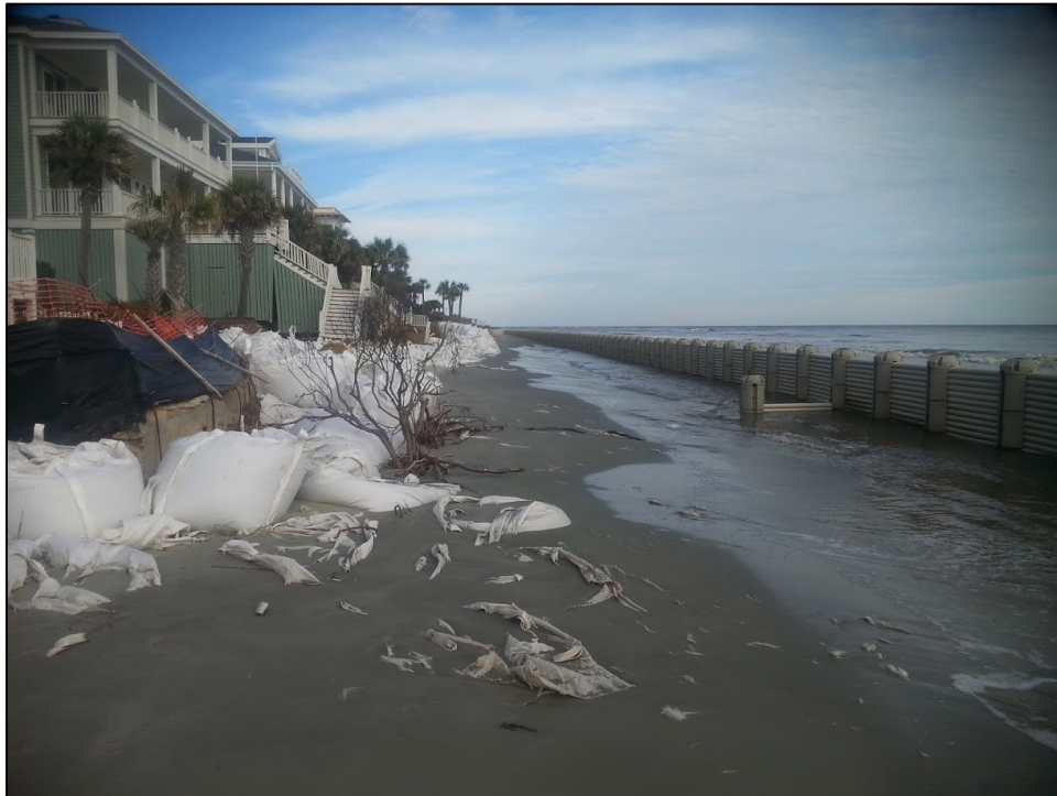
Figure 14. Experimental erosion control structure installed at land-ocean interface at Isle of Palms, S.C. with partially damaged sandbags behind the structure. Photo: NCDCM, 2015
