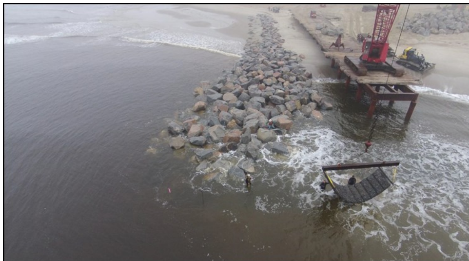
Figure 10. Terminal groin being installed at the Village of Bald Head Island in 2015. Photo: Village of Bald Head Island, 2015
