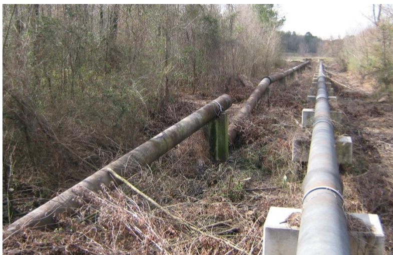
Aerial line collapse due to lack of easement/line maintenance
