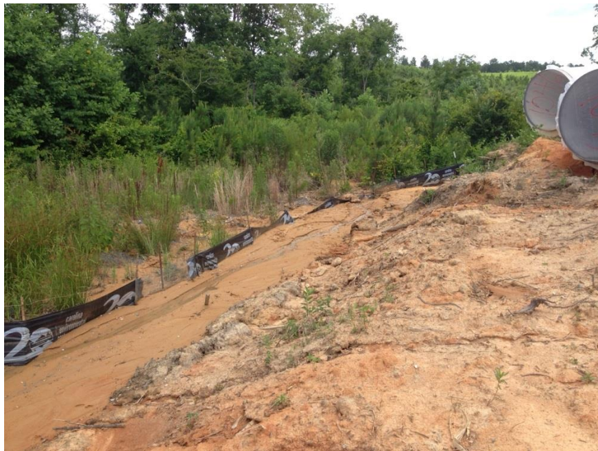
Pipeline project had offsite sediment at multiple locations and times to adjacent property and streams due to poor site management and benched staging of pipe that was not shown on the approved plan.
