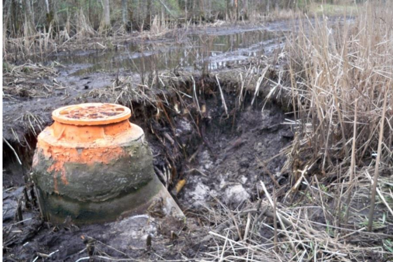
Sewage line interceptor failure and replacement area
