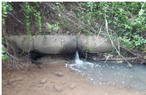
Joint separation from exposed line causing direct discharge to stream
