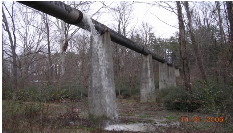
Aerial line failure
