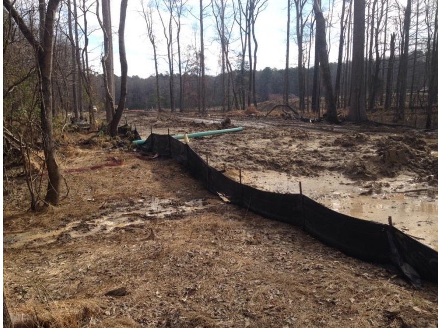
Perimeter silt fence was breached by contractor in effort to dewater the site, resulting in offsite sedimentation.
