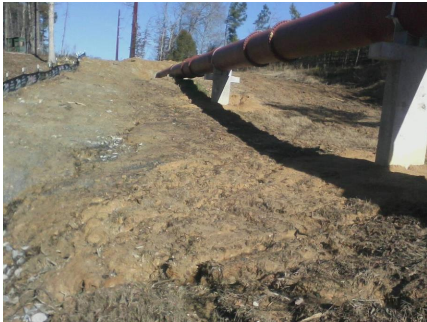
Upstream runoff, poor site management, and lack of groundcover at this aerial utility crossing contributed to offsite sedimentation.
