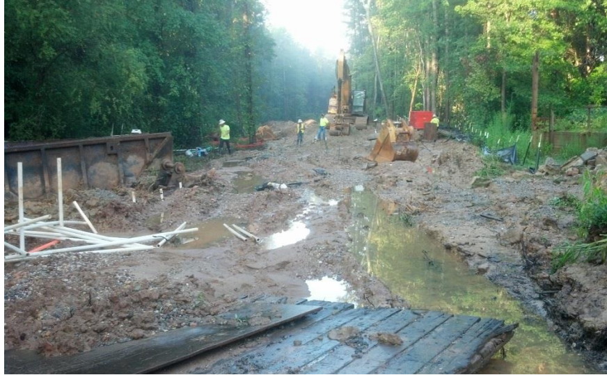
Flooding of project area due to adjacent streams delayed establishment of groundcover, construction, and led to sediment being deposited offsite.
