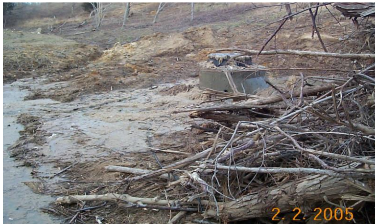
Sewage overflowing from manhole due to line failure
