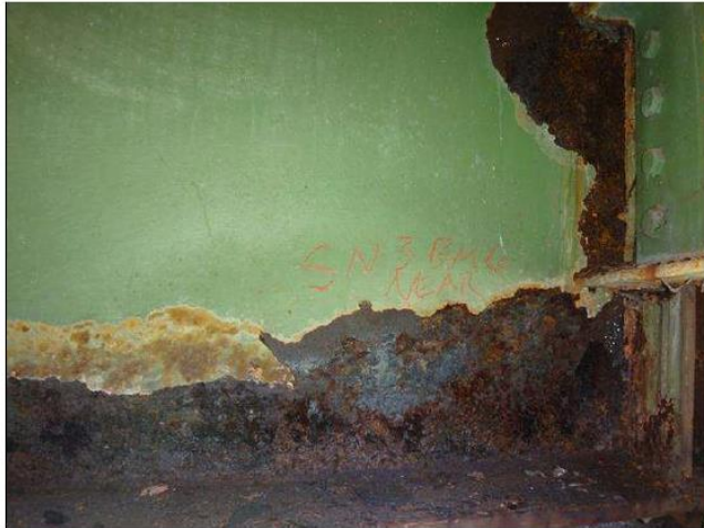
Span 3 Beam 6: [PM] at near half, active corrosion with section loss, at bottom flange [16ft x up to full width - loss<1/16in], at web [16ft x up to full height - avg rem 7/16in], at web stiffener [up to full height x full width - loss<1/16in]
