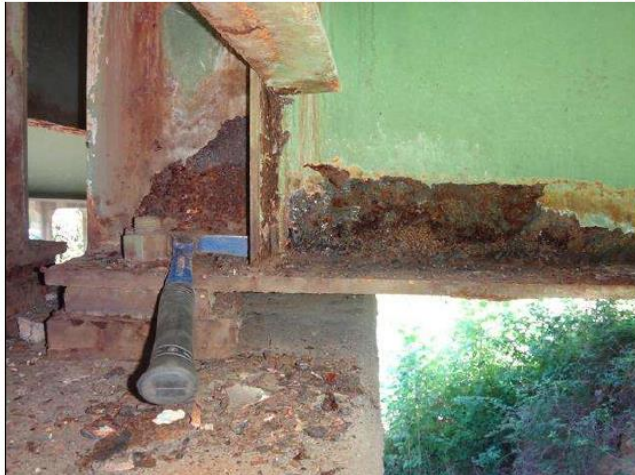
Span 3 Beam 5: at near end, active corrosion with section loss, at bottom flange [6ft x full width - loss<1/16in], at web [6ft x up to full height - avg rem 5/8in], at web stiffener [full height x full width - loss<1/16in]
