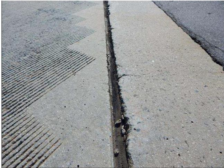
Expansion Joint : SPAN (3) FAR JOINT AT ABUTMENT (B) CRACKED AND LEAKING FULL LENGTH ONTO CAP
