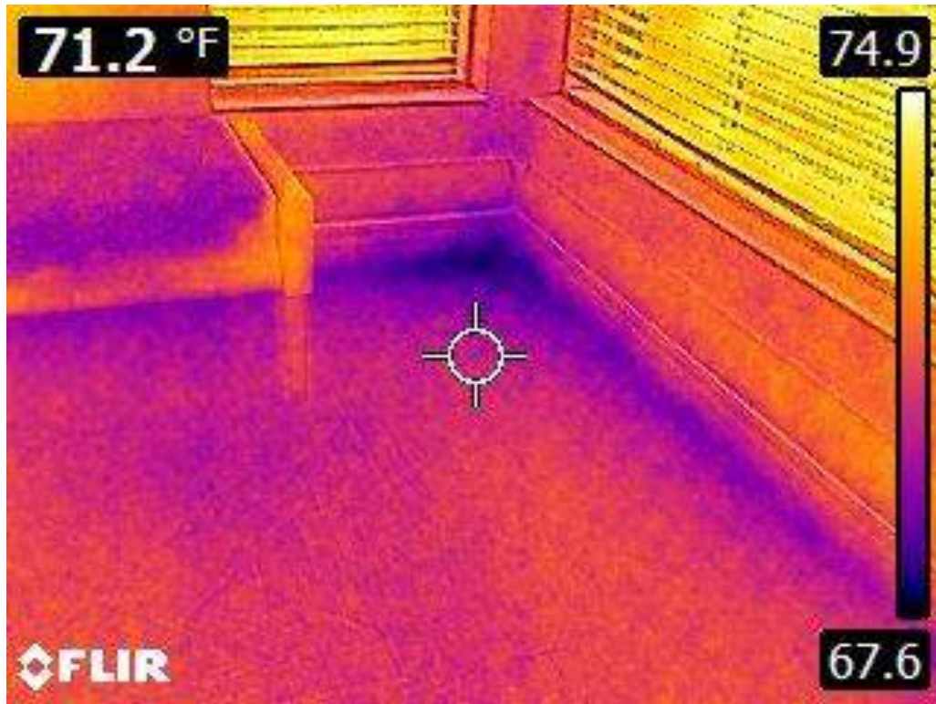
Infrared image of drywall, flooring, and seat cushion with indications of water intrusion.
