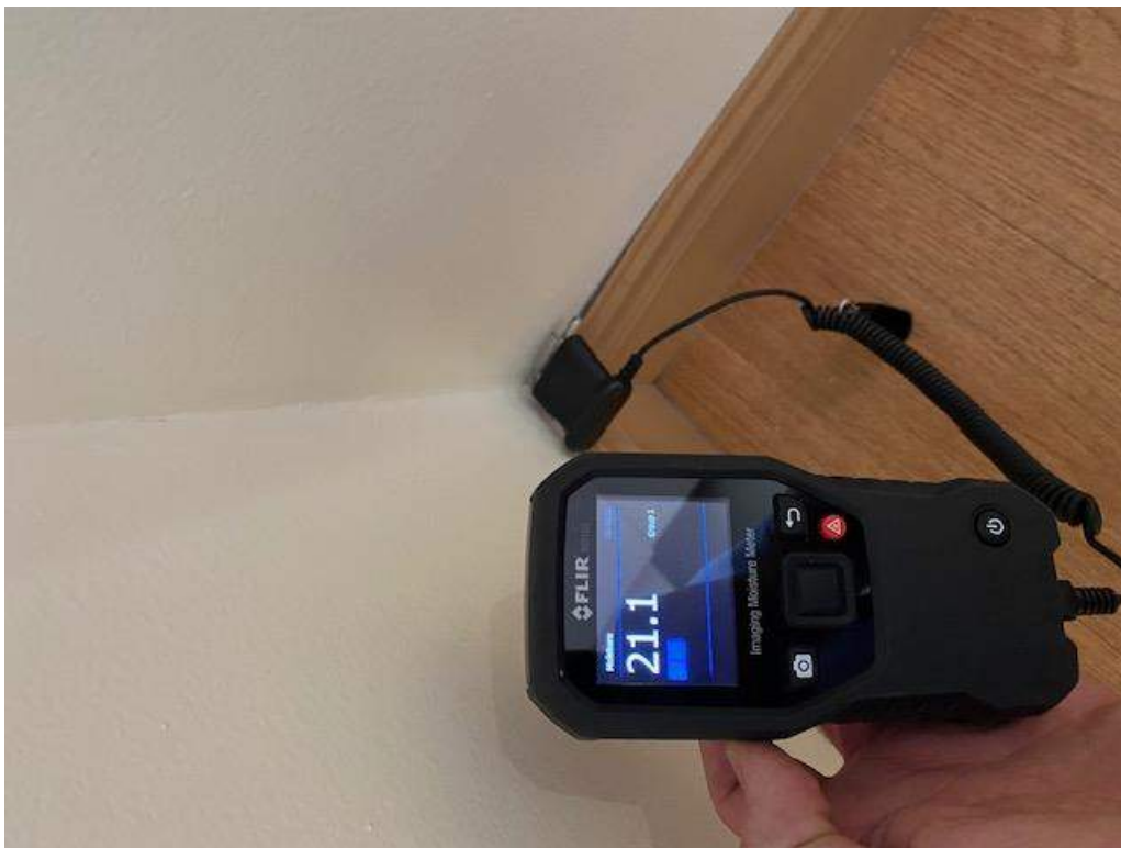
Water intrusion detected in drywall in Core Hall near kitchen.
