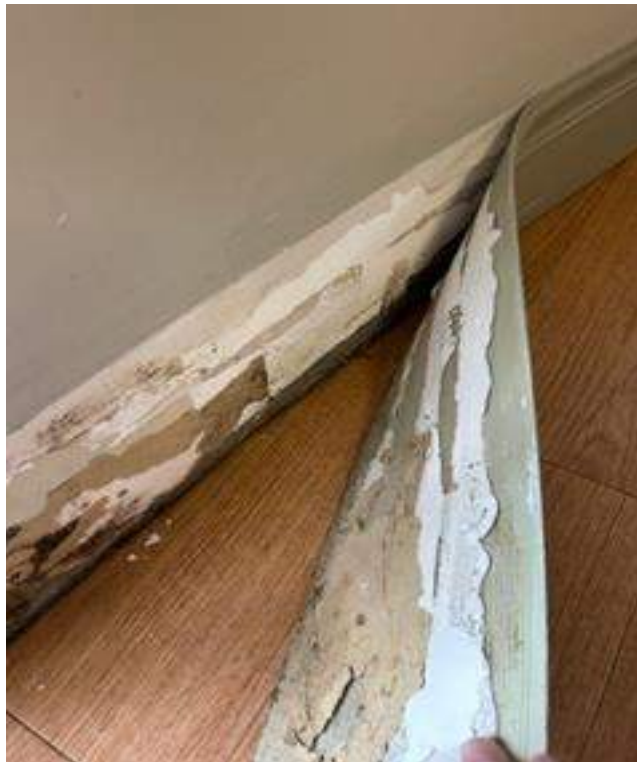
Typical of visible mold growth observed on drywall and cove base throughout the facility.
