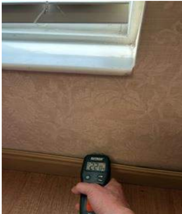
Elevated moisture levels measured in hallway associated with windows throughout the facility.
