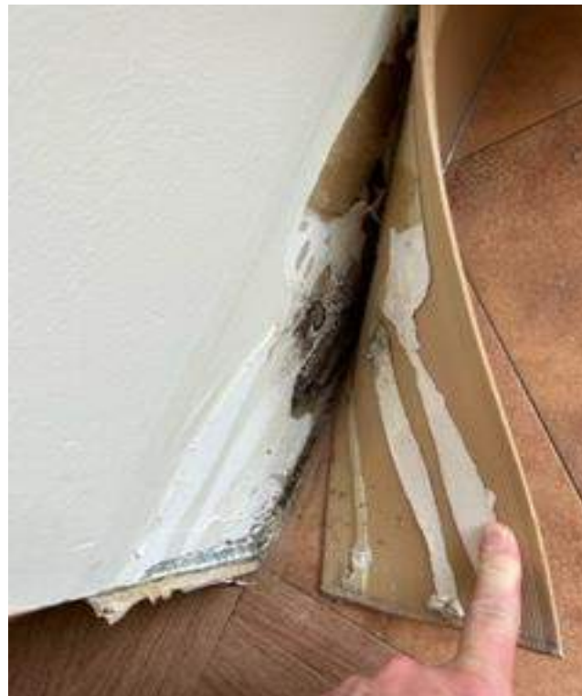
Typical of visible mold growth located behind vinyl cove base throughout the facility.
