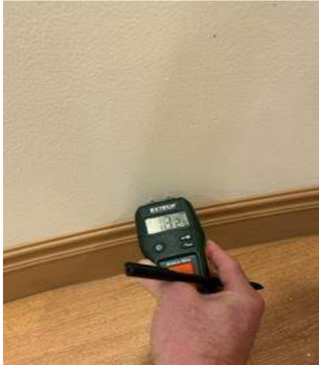
Elevated moisture levels (>16% moisture) measured in the hallway. Elevated moisture levels were observed throughout the facility.
