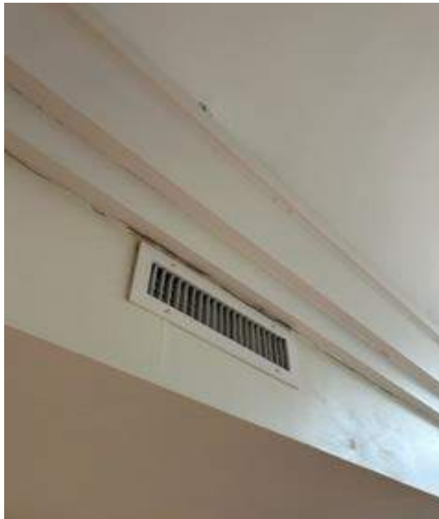
Typical of visible mold growth observed on supply diffusers throughout the facility.
