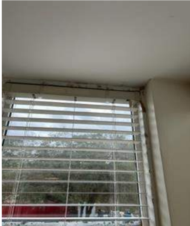
Visible water damage observed associated with window.
