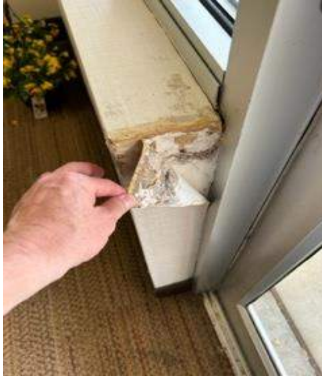
Visible mold growth behind wallcoverings at exterior windows and doors.
