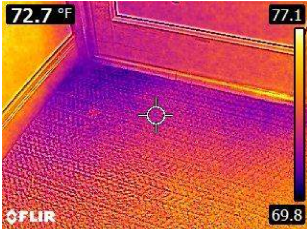
Infrared image of drywall and flooring with indications of water intrusion.
