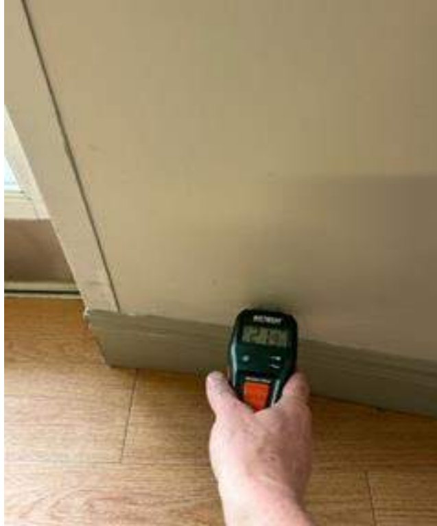
Typical of elevated moisture readings associated with entrance doors and lower walls throughout the facility.
