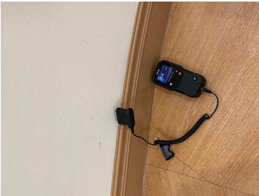
Water intrusion detected drywall in Core Hall near Bravo Wing.
