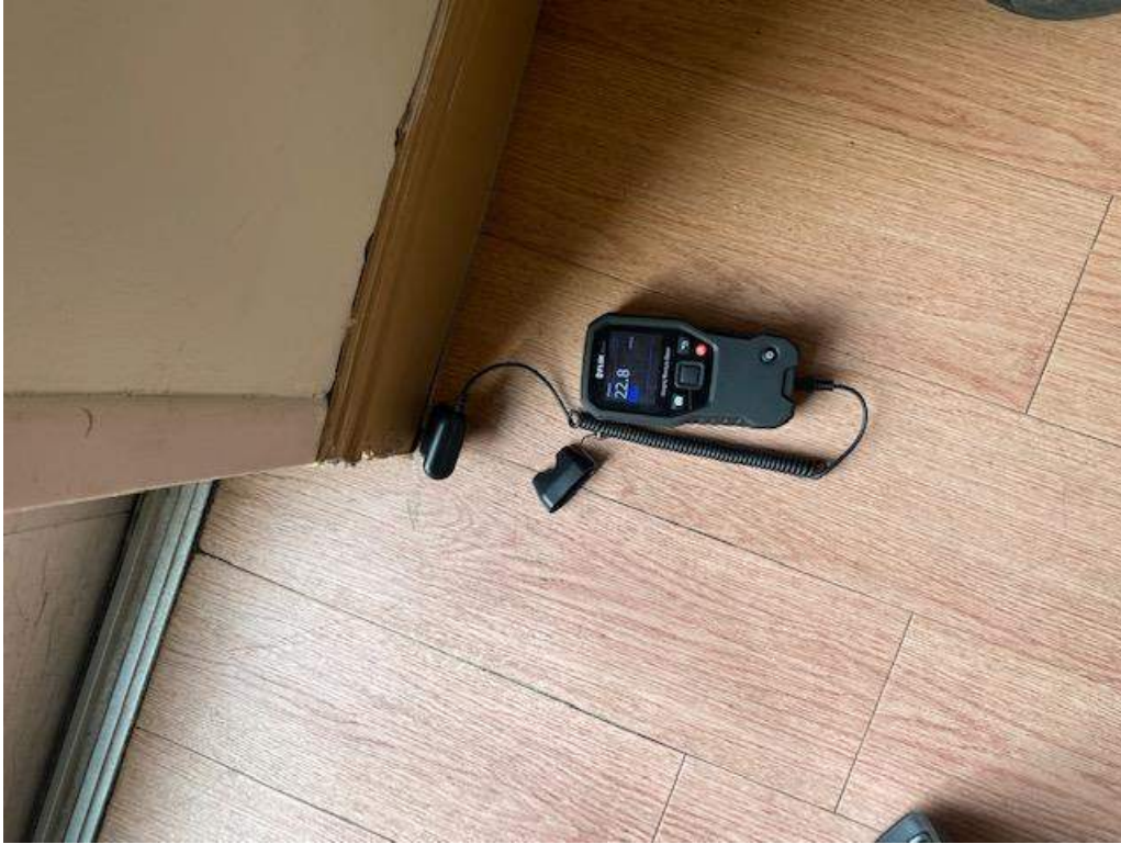
Water intrusion detected under flooring in Core Hall near door.
