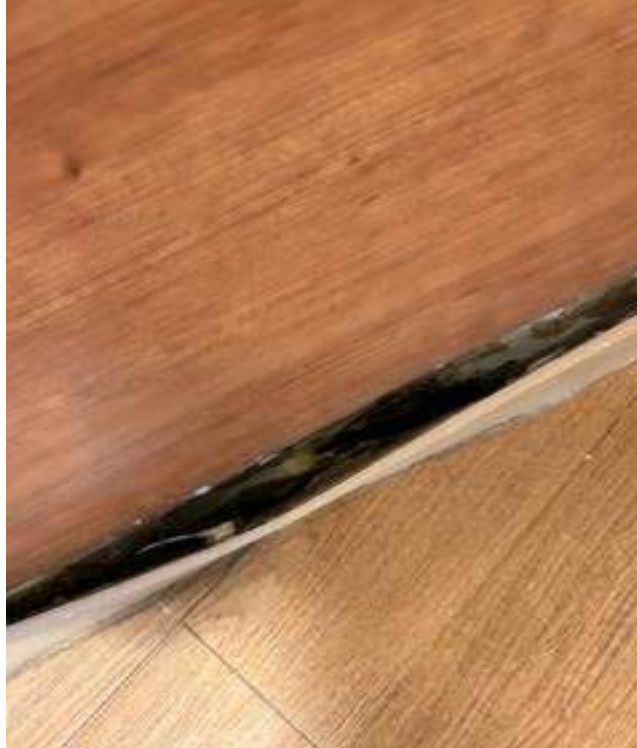
Visible mold growth behind cove base at kitchen hallway. Sample VET-S-01
