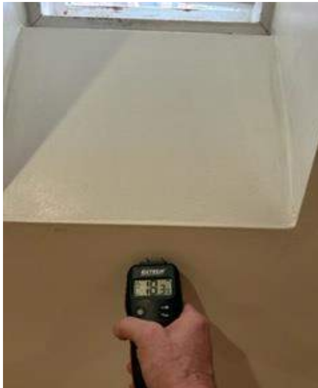
Elevated moisture levels (>16% moisture) measured in the hallway associated with windows throughout the facility.
