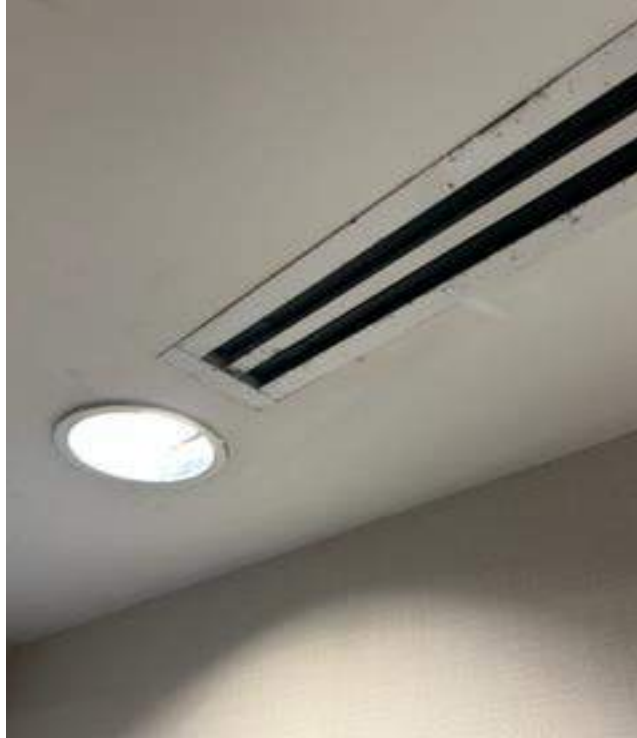
Typical of visible mold growth observed on supply diffusers throughout the facility.
